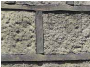
Fig.86: poor quality pointing
